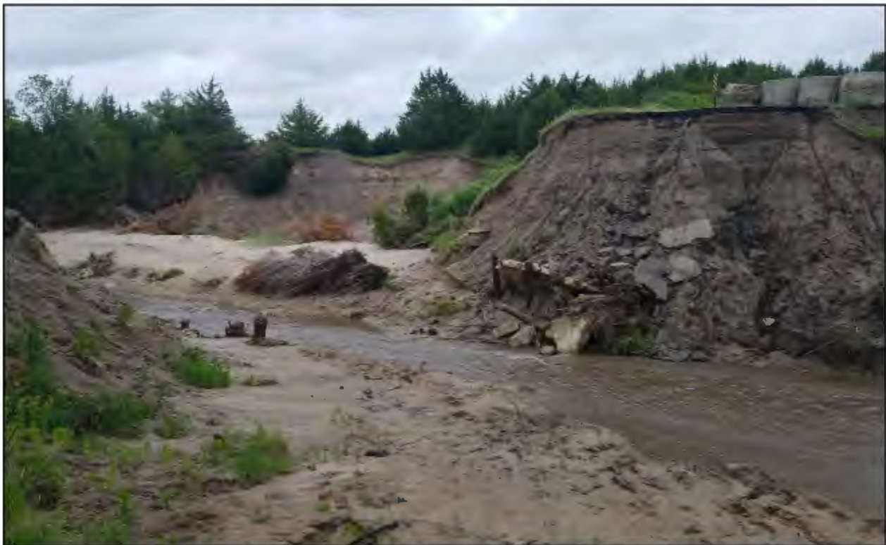
Photograph 2. Looking downstream at the Old Highway 7 failure that occurred in 2019 (FYRA, 2020)
